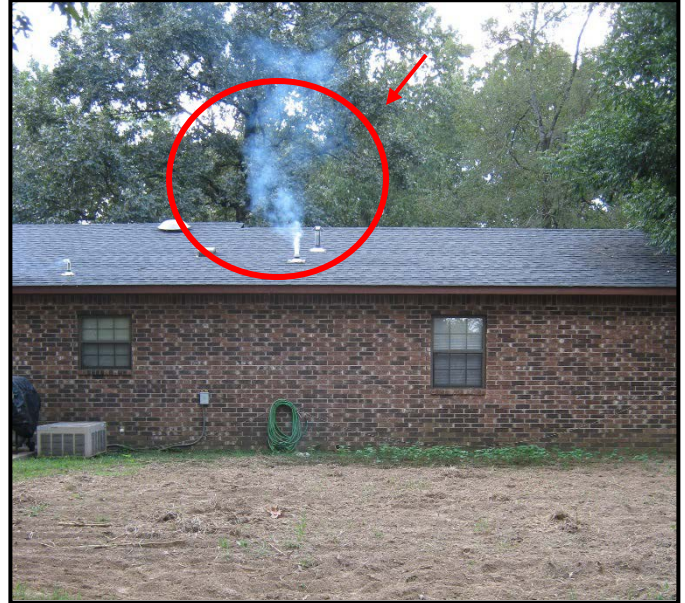
Smoke may exit from the vent pipe on top of each residence during smoke testing.
